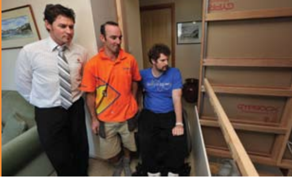
Joe O'Byrne, Nigel Curran and Callum Davis inspect works during the installation of a lift at Callum's Launceston home.
